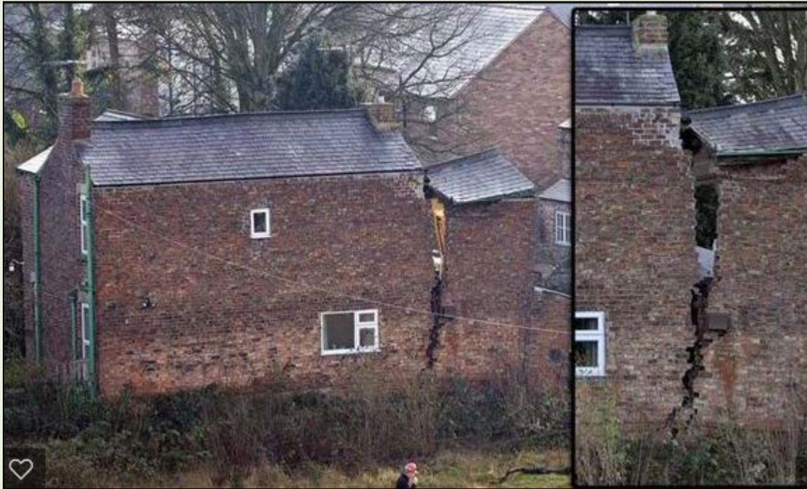
Fracture developed in house above a sinkhole
